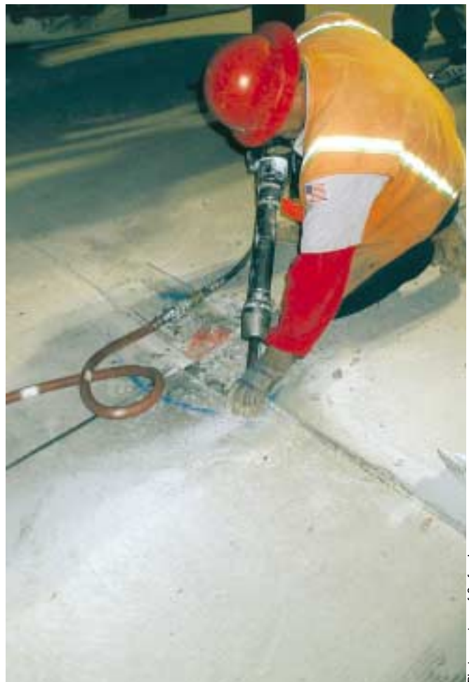
Hand work with a pneumatic hammer is needed to prepare this smaller spill for repair.
