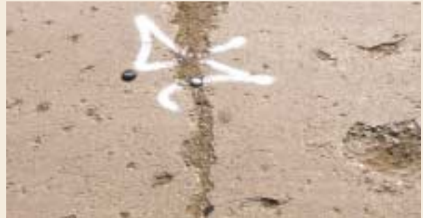
This failed concrete pavement joint is packed with debris and incompressible matter that will cause great damage in freeze-thaw cycles.
