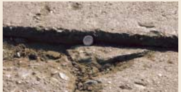
A subgrade failure caused this concrete slab fault from below.
