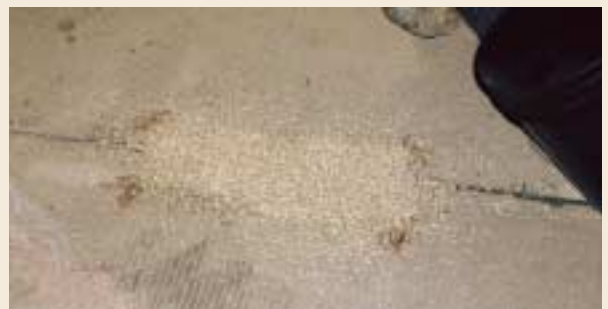
Limited spalling at failed joints may be repaired using ultra-fast proprietary patching compounds- in this case, TechCrete.
